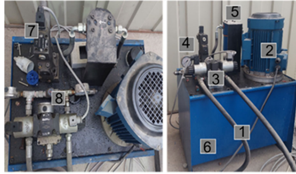
Figure 3. Hydraulic actuator components.
